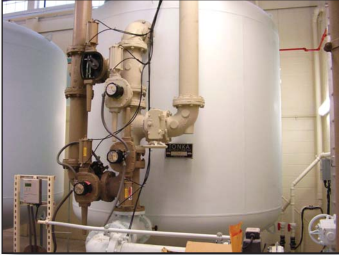
Four Tonka Anion Exchange units each treating up to 400 gpm
