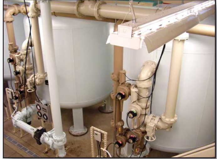
Tonka's system responsibility includes anion exchange vessels, resin, valves, facepiping, instrumentation, brinemaker, control descriptions, and softener system
