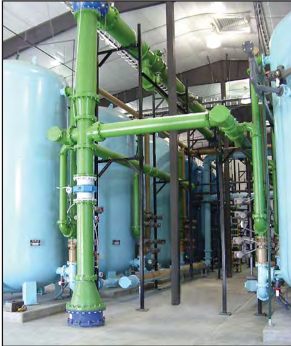
A computerized (PLC) control system operates 6 cation vessels and 6 anion vessels.
