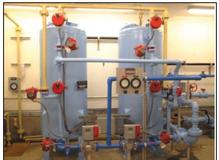
Two Tonka Ion Exchange vessels remove nitrates, providing quality water for Boone residents.
