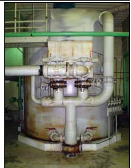
Aurora, MN – Tonka's Simul-Wash™ Serial No. 0001, circa 1979 and new filter installed 2009 (top)
