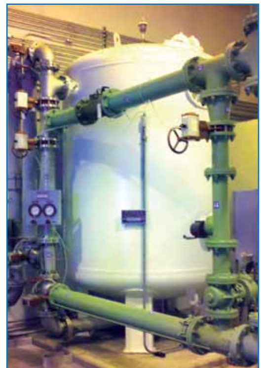
Warm Springs, Georgia Water Treatment Vessels
