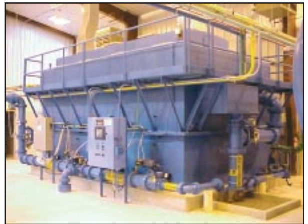
Dualator® III Iron and Manganese Removal System Country Estates, Wisconsin
